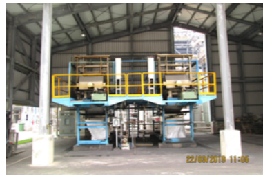
Catalyst recovery pretreatment unit
