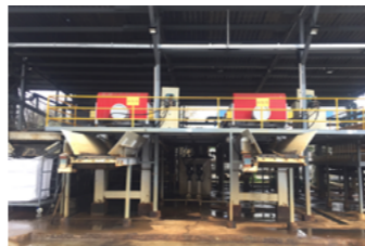
Installation of 2 sludge dryers with plate and frame filter press at FEDZ
