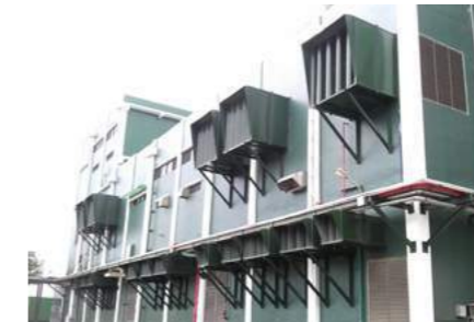
A muffler installed for the exhaust port
